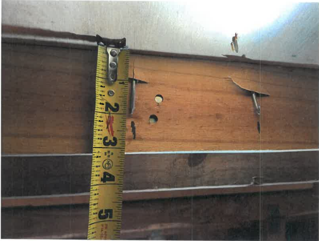
Figure 3 – Sheathing Fastener Size 8d Confirmed (Typical)
